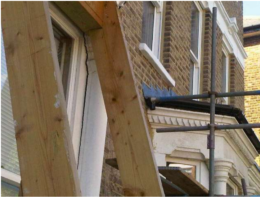
Cracked window frame and emergency structural support at 92 South Hill Park, caused by basement development next door
