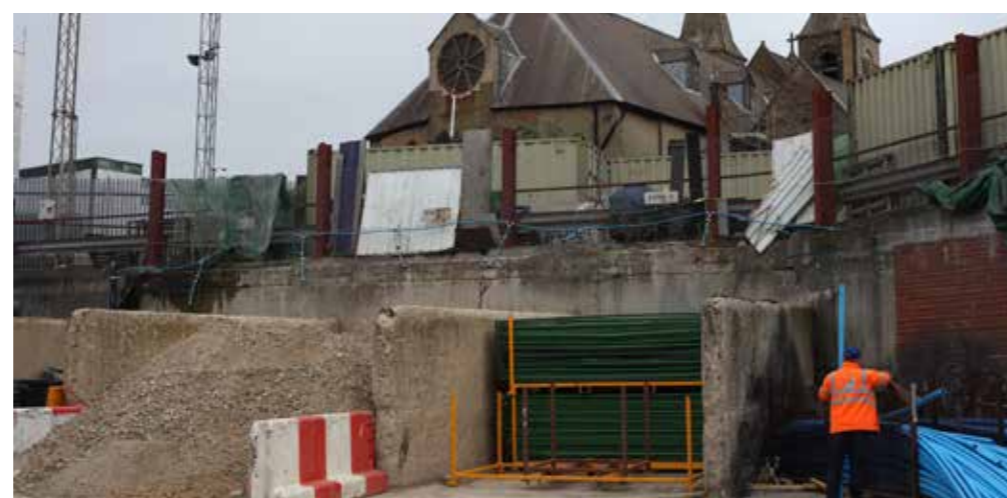
Significant level changes
