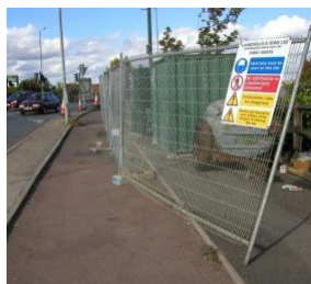
Building materials left on cycle track
