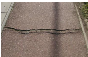
Surface cracking or excessive rutting
