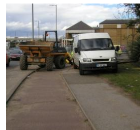
Contractors obstructing cycle route
