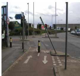
Damaged sign obstructing cycle track
