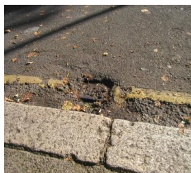
Worn/smooth manhole covers
